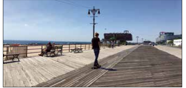
There are broken planks and exposed nails on many other sections of the Boardwalk besides the plywood-covered part.
