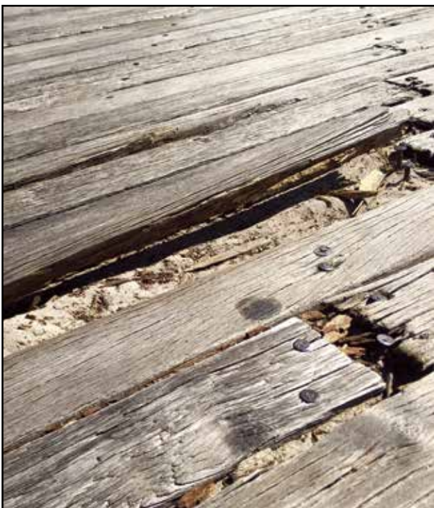
So many spots on the Coney Island Boardwalk need to be repaired.
